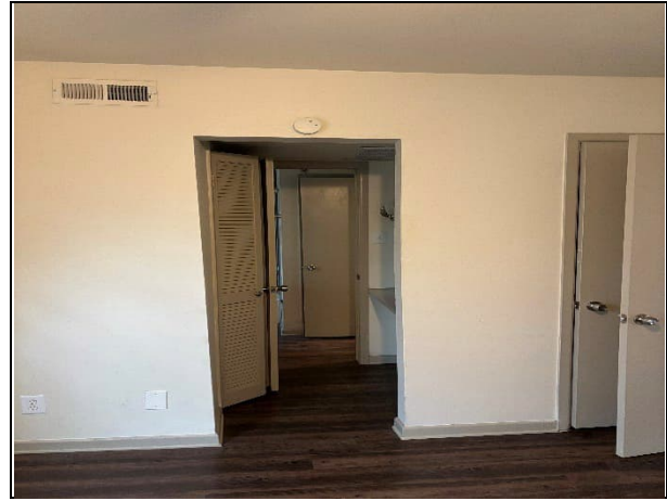
Photo #14 Asbestos containing finished drywall wall with texture (sandy).
