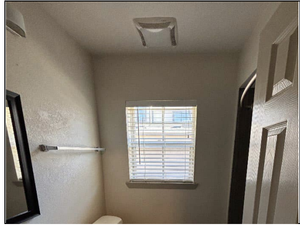
Photo #8 Asbestos-containing finished drywall wall with texture (orange peel).
