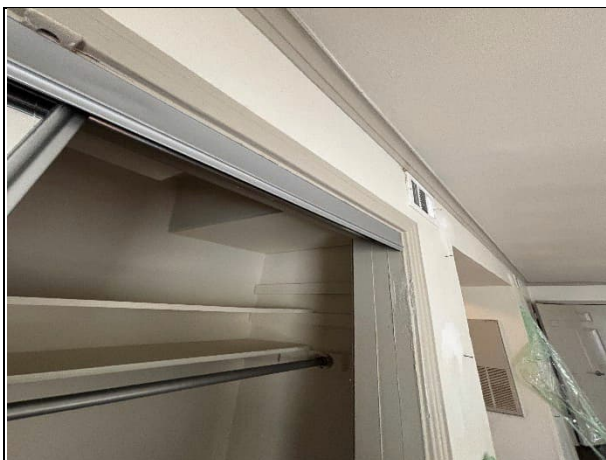
Photo #11 Asbestos containing finished drywall ceiling with texture (semi-smooth).
