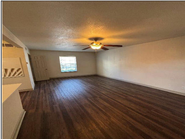
Photo #9 Asbestos containing finished drywall ceiling with texture (orange peel).
