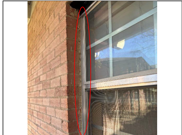
Photo #4 View of asbestos-containing exterior window frame sealant.
