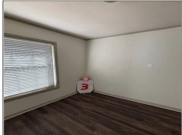
Photo #10 Asbestos containing finished drywall wall with texture (semi-smooth).
