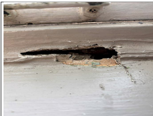
Photo #5 View of asbestos-containing interior window frame sealant.
