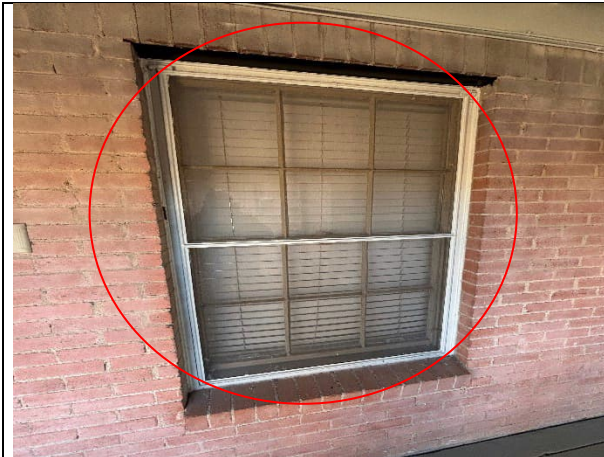
Photo #3 View of asbestos-containing exterior window glazing compound.
