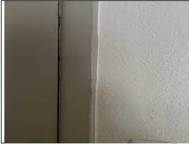
Photo #7 View of asbestos-containing interior door frame sealant.
