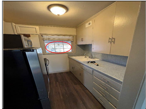
Photo #2 View of window with asbestos-containing interior window glazing compound.
