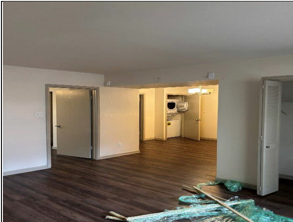
Photo #15 Asbestos containing finished drywall ceiling with texture (sandy).
