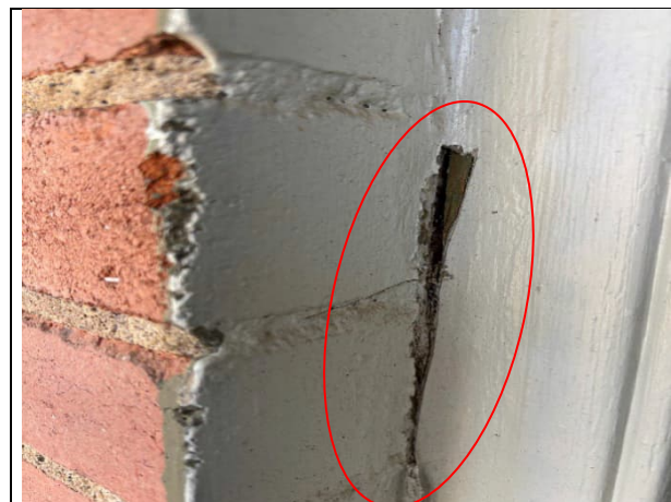
Photo #6 View of asbestos-containing exterior door frame sealant.
